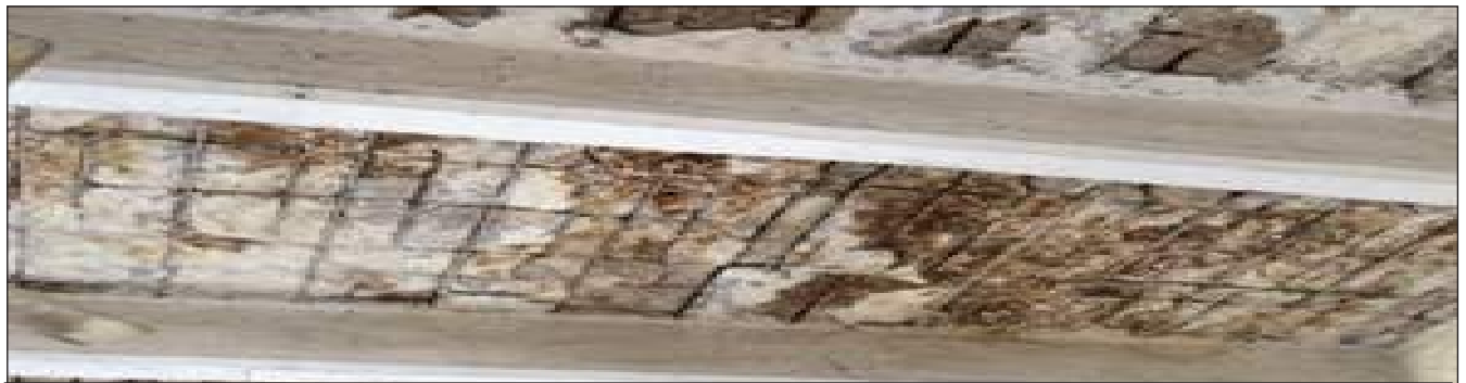
The barracks of Central Prison Sukkur were in dilapidated condition.
